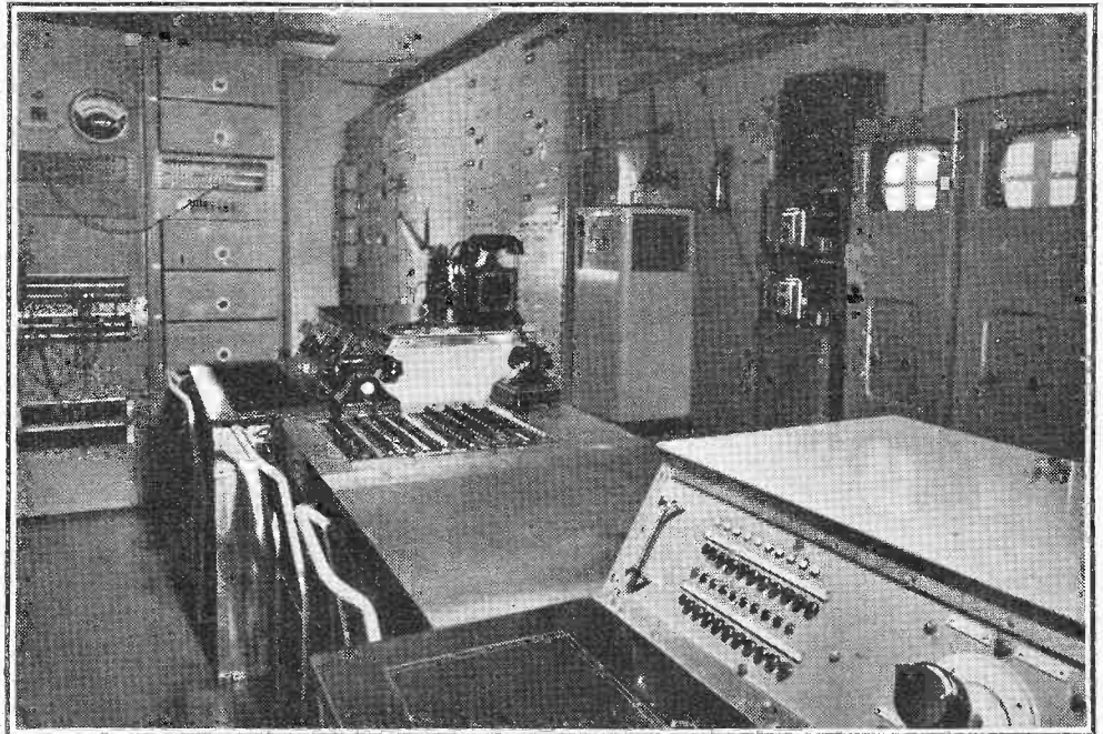
The central control room of the London television station which handles the outputs of the two studios as well as those coming from the O.B. vans whether by cable or radio link. The vision mixing desk and monitor are on the right with the sound mixing desk on the left and the production manager's desk in the centre.
